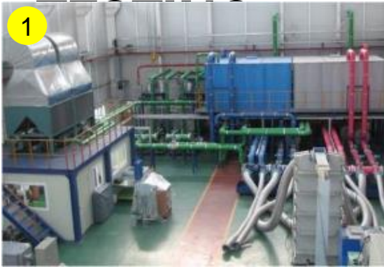
Water to Water test facility
