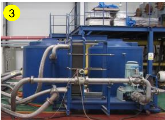
Seawater supply facility
