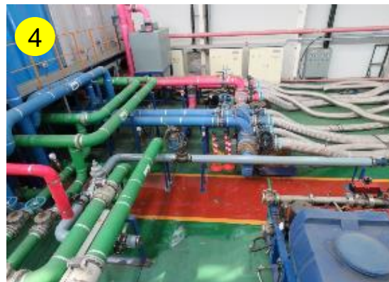
Steam supply facility
